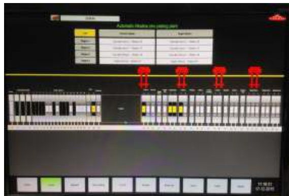
SCADA - Surface Treatment Plant
