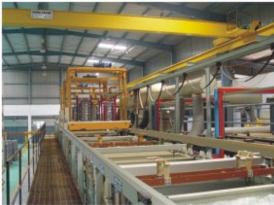
Fully automatic PLC controlled plating system
