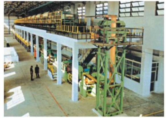
Continuous plating lines for plating of strips, tube wires etc.
