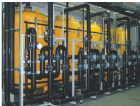
Ion Exchanger Re-circulation System
