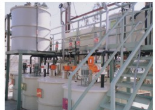
Fully Automatic ETP Plant
